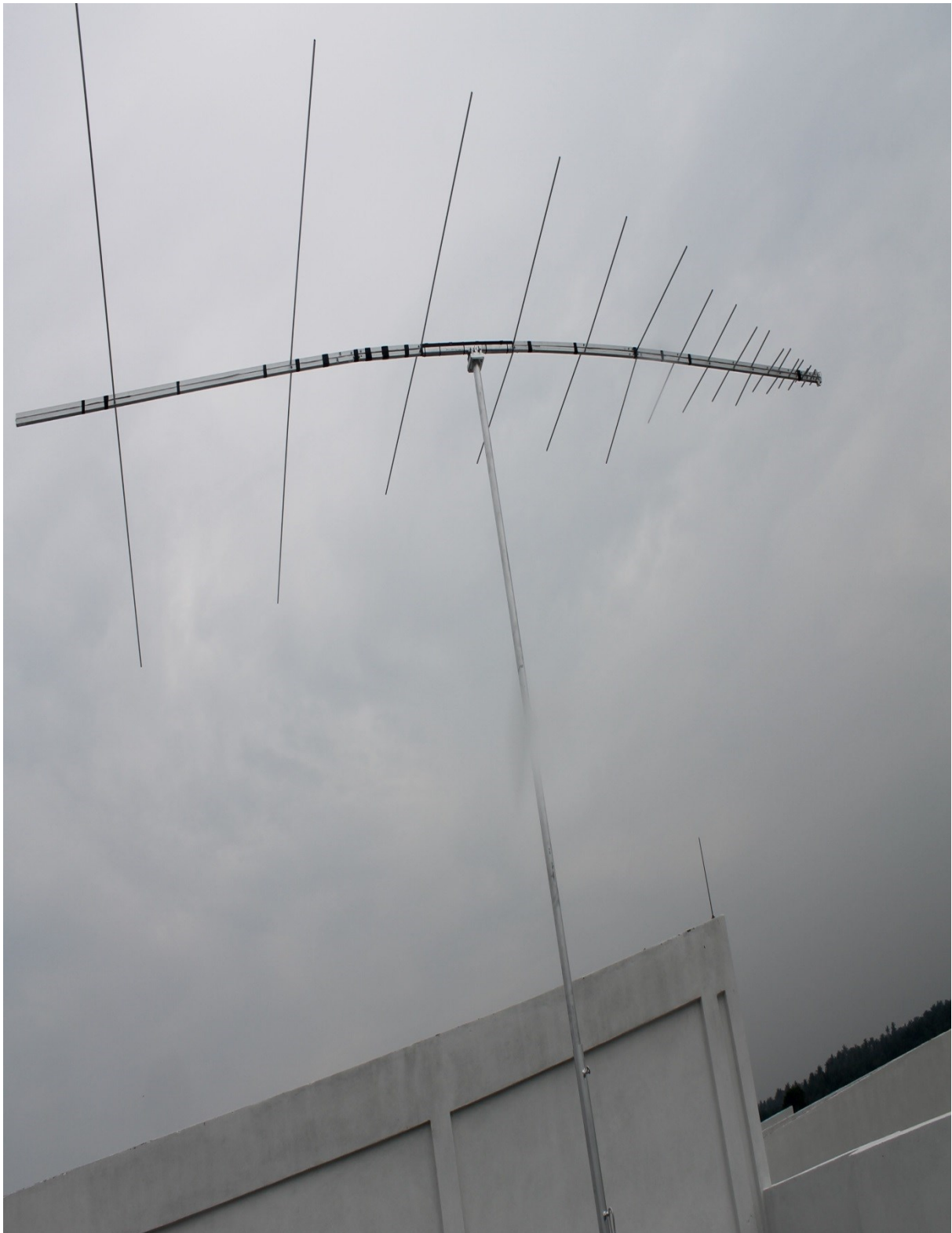
Figure 3. The installation of 5.5 meters Log Periodic Dipole Antenna at the National Space Centre Banting, Selangor Malaysia.
